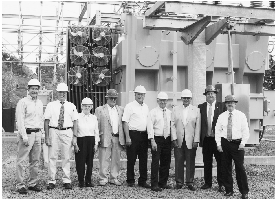
Wellsboro Electric officials stand in front of the new Buena Vista Street substation transformer. Shown are, from left, WECO President and CEO Craig Eccher and board members Steve Sliwinski, Barbara Seeley, James Luce, Al Calkins, Erick Coolidge, board Chairman Tom Rudy, Kevin Barrett and Ron Gilbert.
